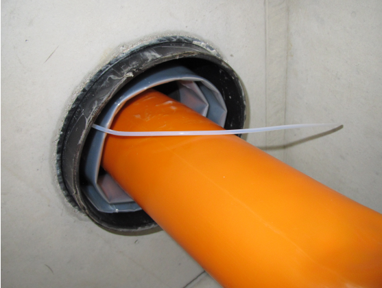
Combined installation of the TE connectivity ADE / TDUX in the KKR 110
